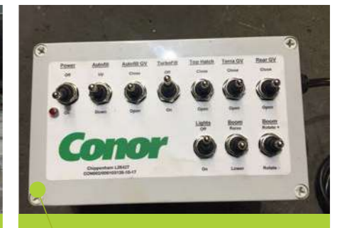
Electronic control box
